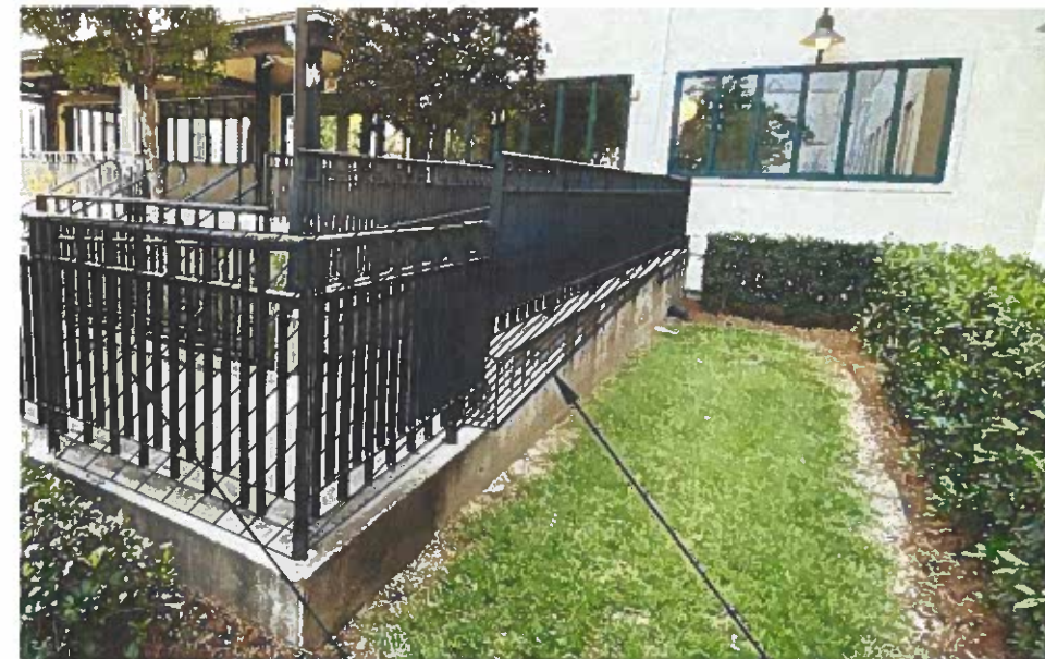
GUARDRAIL TO BE REMOVED. SEE SHEET C-008 FOR NEW GUARDRAIL CONNECTION TO EXISTING LANDING
