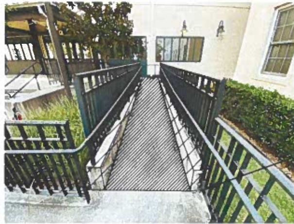
EXISTING 8" THICK WALLS ON BOTH SIDES OF RAMP TO BE CHIPPED TO 3" BELOW THE BASE OF RAMP SURFACE AND FILLED BACK WITH CONCRETE FLUSH WITH EXISTING RAMP.
