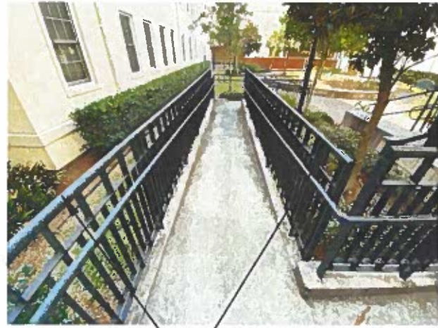
EXISTING GUARDRAIL AND HANDRAIL TO BE REMOVED AND REPLACED WITH NEW GUARDRAIL AND HANDRAIL
